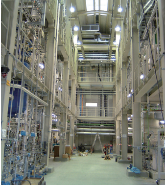
The Direct Devolatilization process was implemented on a semi-industrial scale at the Fraunhofer Gesellschaft in Germany.
